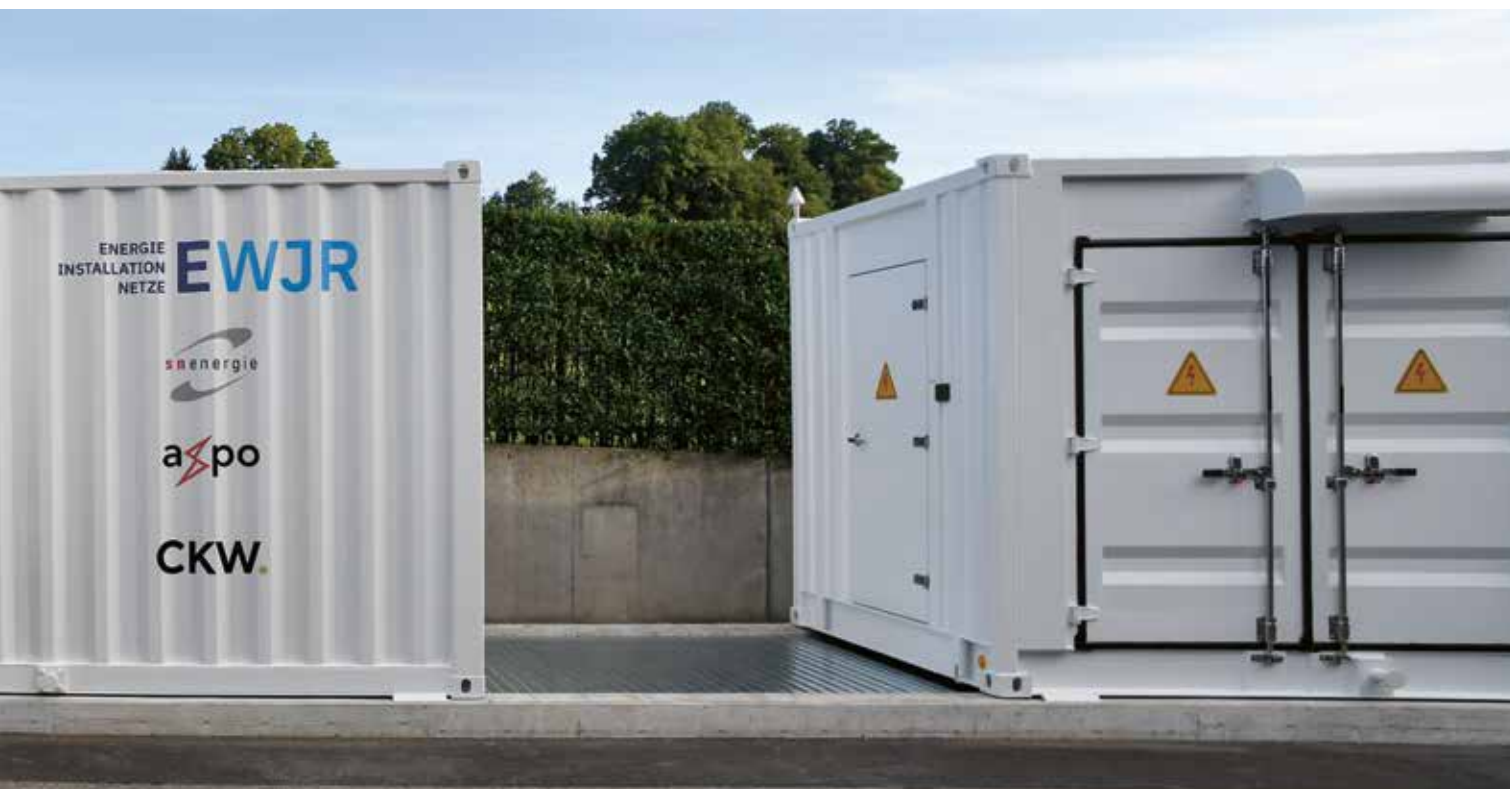
Axpo battery storage system 2 MW / 2.17 MWh, completed 2019, end customer Elektrizitätswerk Jona-Rapperswil AG (EWJR), Switzerland
