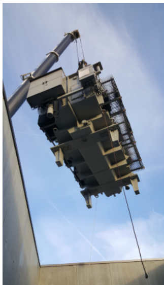
The transformers weighing 42 to 71 tonnes are lowered into the substation by crane through an opening in the roof.
