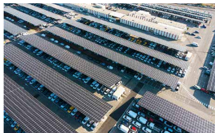
Urbasolar’s photovoltaic system, which also provides shade for cars, in Bouches-du-Rhône, France.
